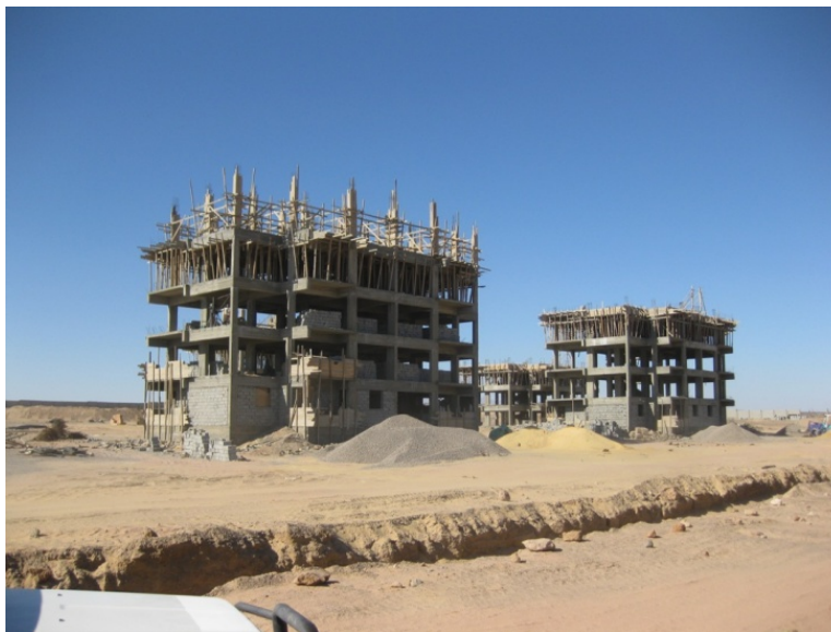
Figure 1.12: Example for service building construction for two wind farms of about 200 MW each
