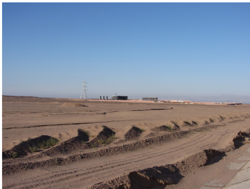
Figure 1.10: Suez Gulf (500 MVA) 500 / 220 kV substation
