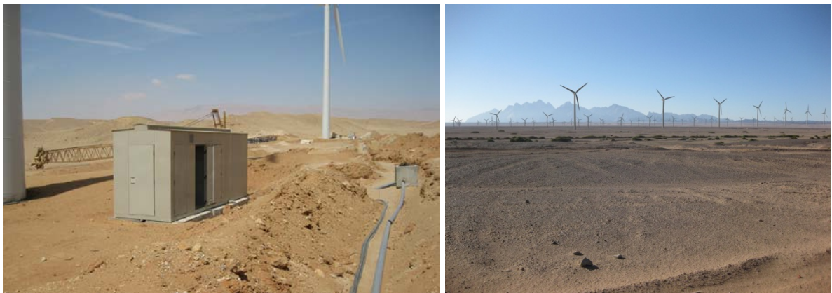
Figure 0.2: Typical Arrangement of kiosks and cabling at a wind turbine (left) and visualization of a typical wind farm in a desert area at the Red Sea coast
