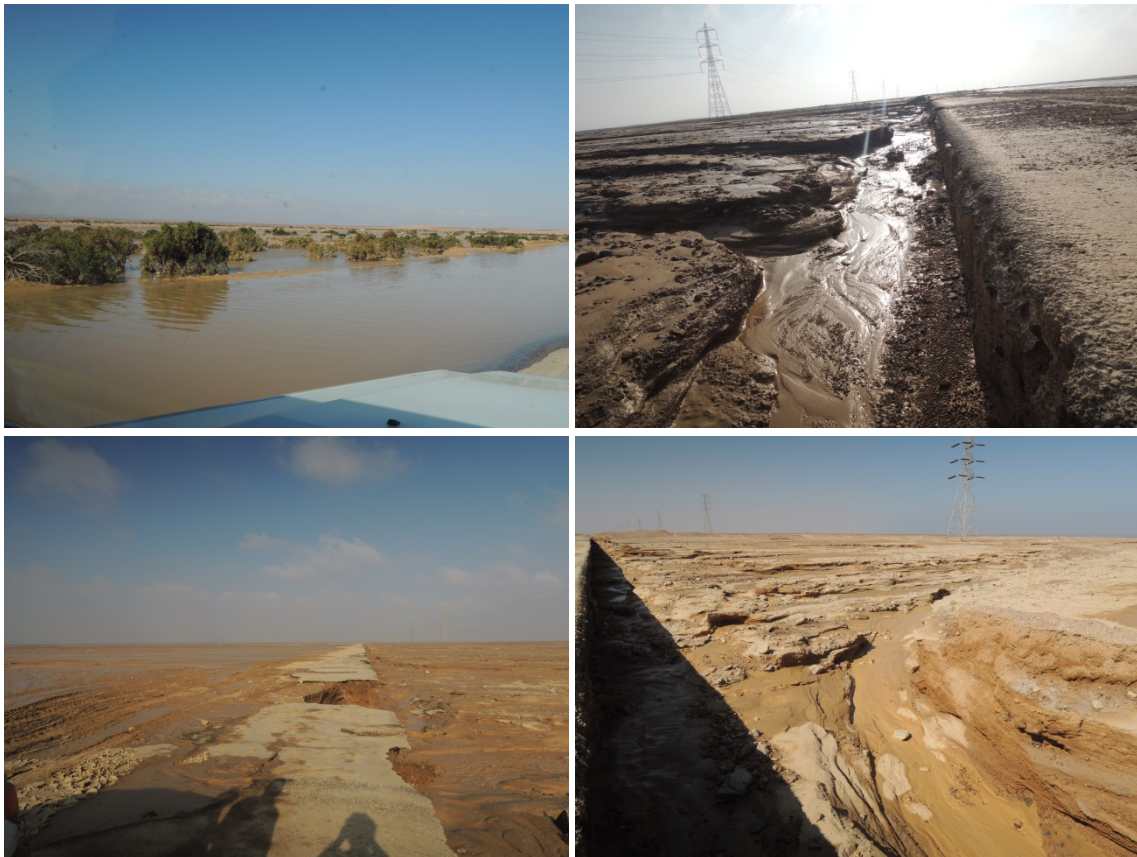
Figure 4.6: Results of the heavy flash floods occurred in late October 2016 in the project area
